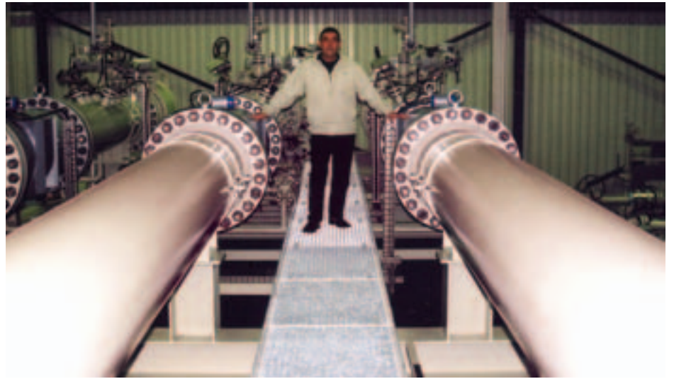
Zero maintenance and lowest cost of ownership. Triple bank of ultrasonic flowmeters
